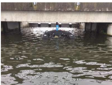
OLOID Type 400 with flow direction to the dam shutter
